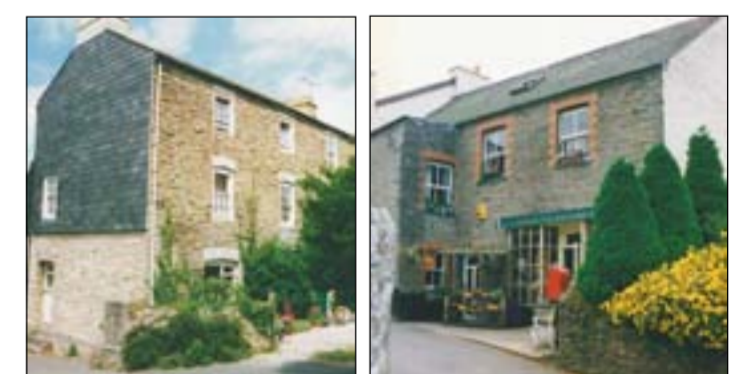
Only a handful of historic buildings reveal the use of brick, mainly as a window, door or corner dressing (above right). Slate as a wall cladding is rare too, although the prominence of the elevations so treated create a different impression (above left)
