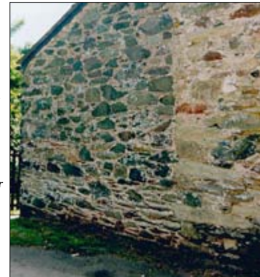
Locally sourced stone is the dominant walling material. It comes in a wide range of colours and types which not only create visual interest they promote other interests too, here giving clues about the age and development of a building
